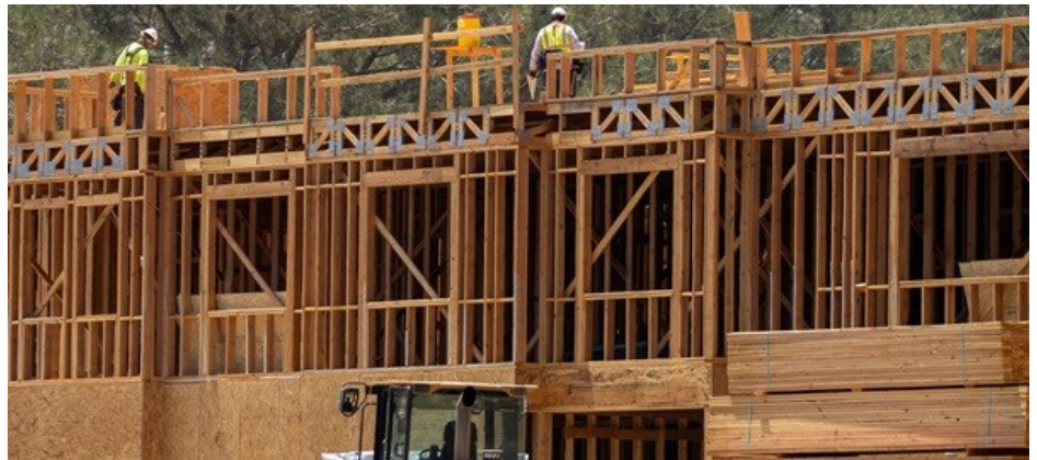
Construction workers on the job at a residential project in Encinitas, California, July 30, 2020. REUTERS/Mike Blake
