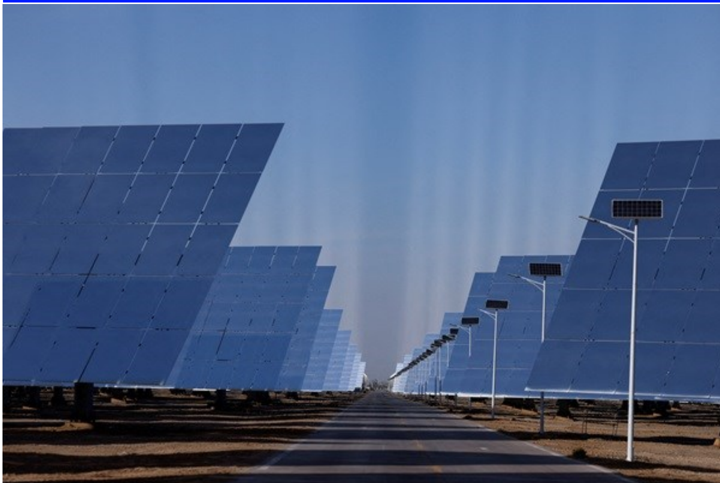
Fields of heliostat mirrors reflect sunlight at the site of Dunhuang Shouhang 100MW Tower Solar Thermal Power Generation Project, during an organised media tour to Dunhuang Photovoltaic Industrial Park, in Gansu province, China, October 16. REUTERS/Tingshu Wang
