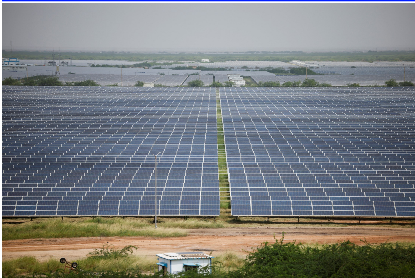
A general view of solar panels at Gujarat Solar Park also called Charanka Solar Park at Patan district in Gujarat, India September 12. REUTERS/Amit Dave
