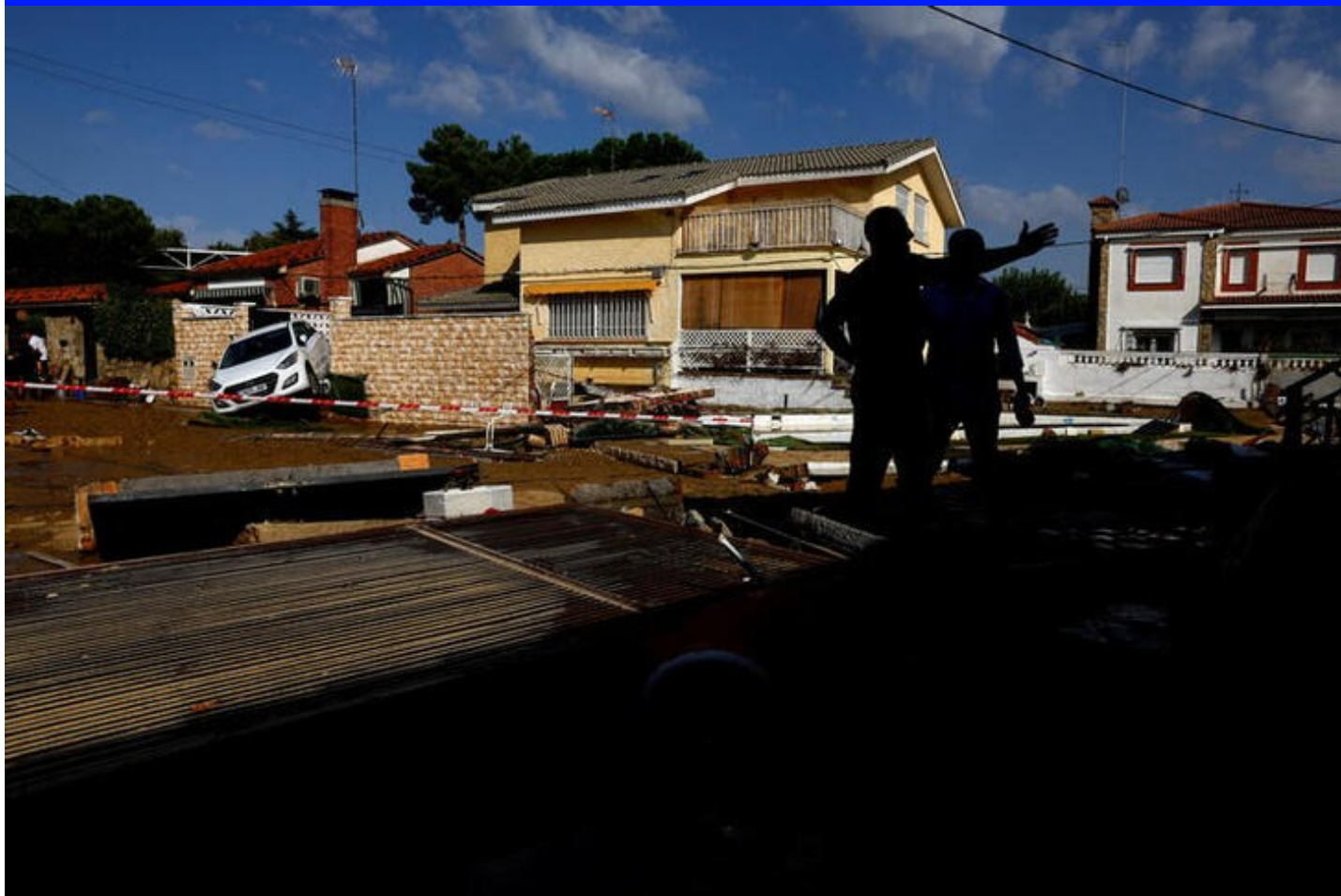
David Fernandez, 52, shows damage on the homes of his parents and their neighbours following heavy rain, in El Alamo, Spain, September 4. REUTERS/Susana Vera
