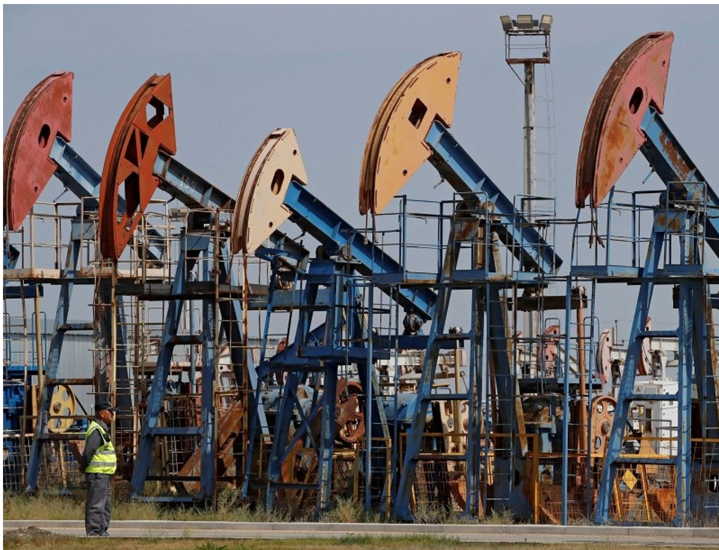
A security guard stands near disused oil pump jacks at the Airankol oil field operated by Caspiy Neft in the Atyrau Region, Kazakhstan August 22. REUTERS/Pavel Mikheyev
