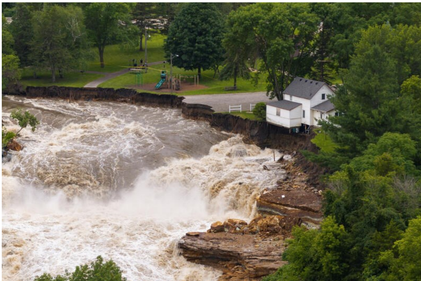
A drone view shows debris accumulating on the Rapidan Dam after torrential rains caused the Blue Earth River to swell, southwest of Mankato, Minnesota, U.S. June 25, 2024. REUTERS/Ben Brewer
