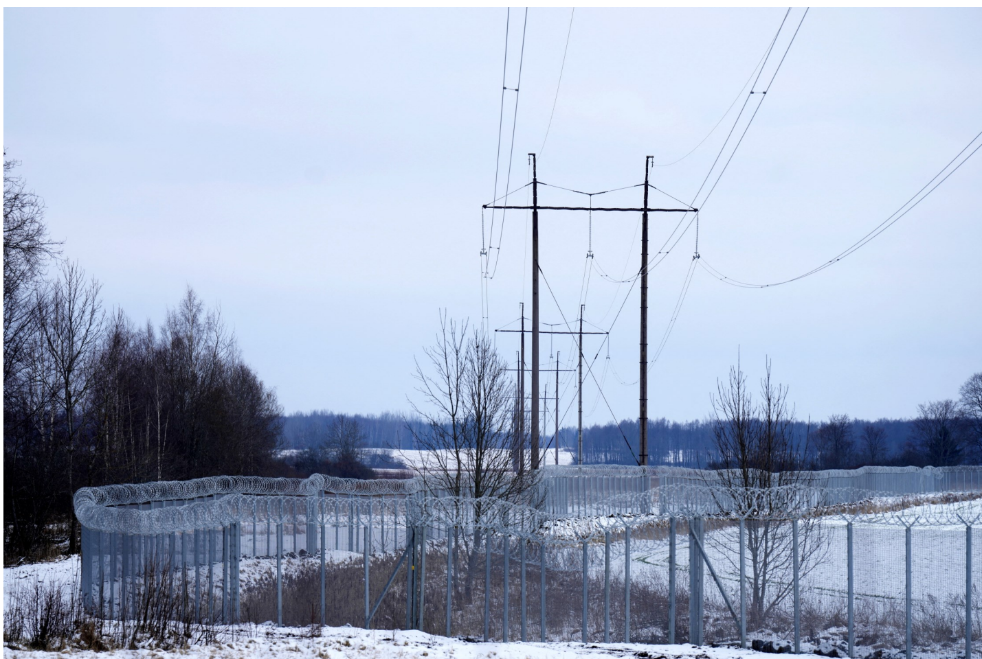
A high voltage line from Russia crosses the border with Russia near Vilaka, Latvia February 8. REUTERS/Ints Kalnins
