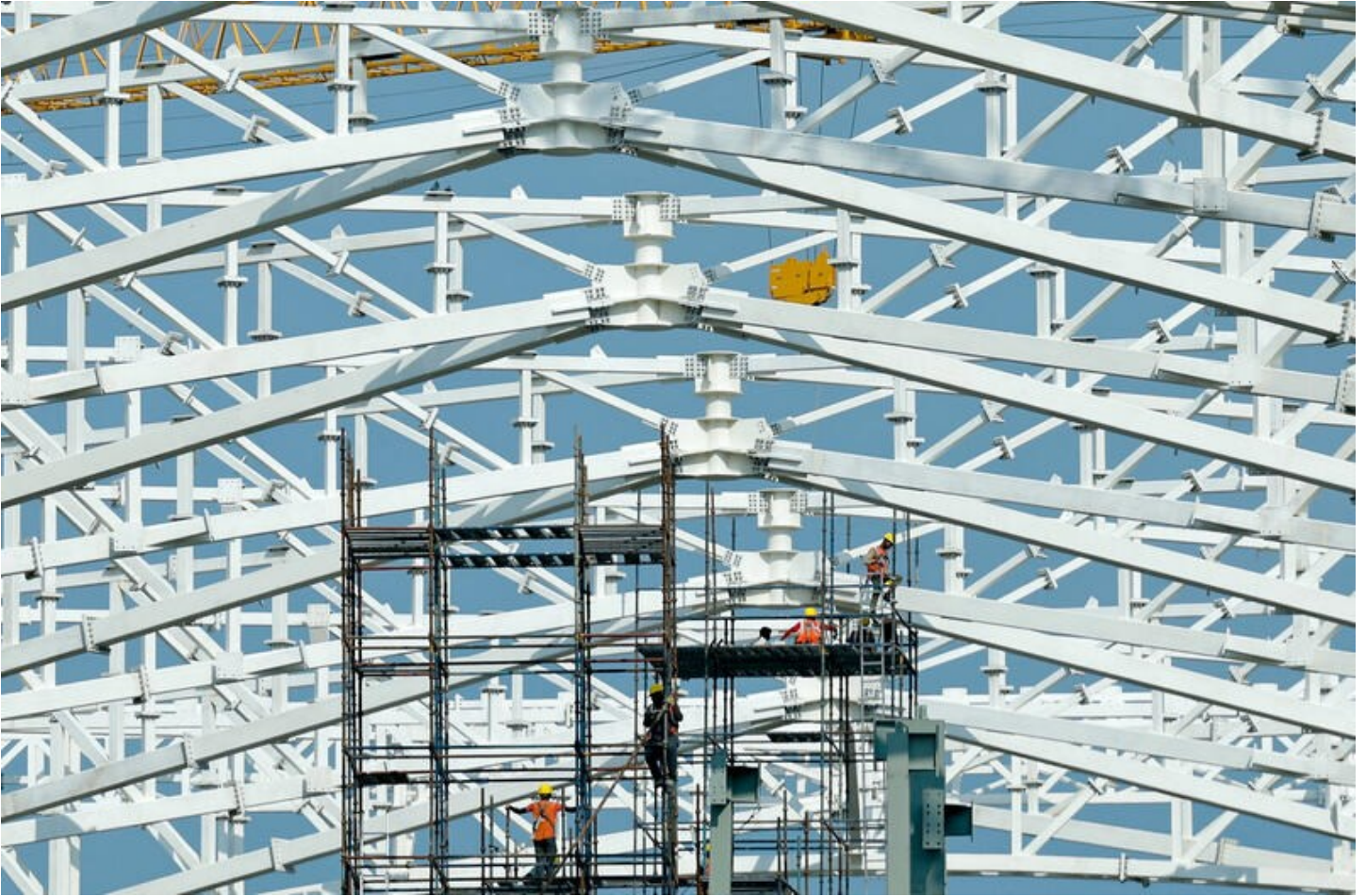
Labourers work at the site of the ongoing construction of Noida International Airport (NIA) during a media visit to the project site, in Noida, August 29. REUTERS/Anushree Fadnavis
